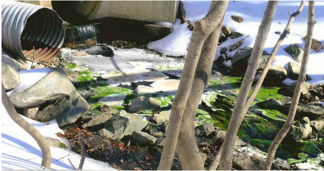
Photo taken on a Crum Creek tributary in winter showing detergent discharge from stormwater outfall and algae in the stream.
