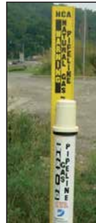
5. HCA marker and cathodic protection test station
