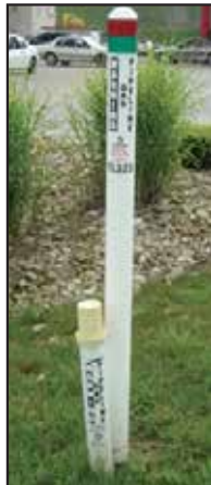
2. Linemarker and cathodic protection test station
