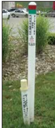
2. Linemarker and cathodic protection test station
