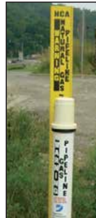
5. HCA marker and cathodic protection test station
