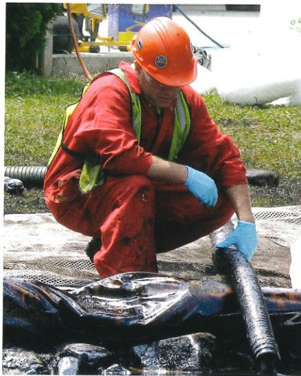
A worker watches water come out of a pipe in Talmadge Creek where booms have been set up to contain an oil spill in Marshall Township, Mich., near the Kalamazoo River. Photo credit: Paul Sancya/ AP/ Shutterstock
