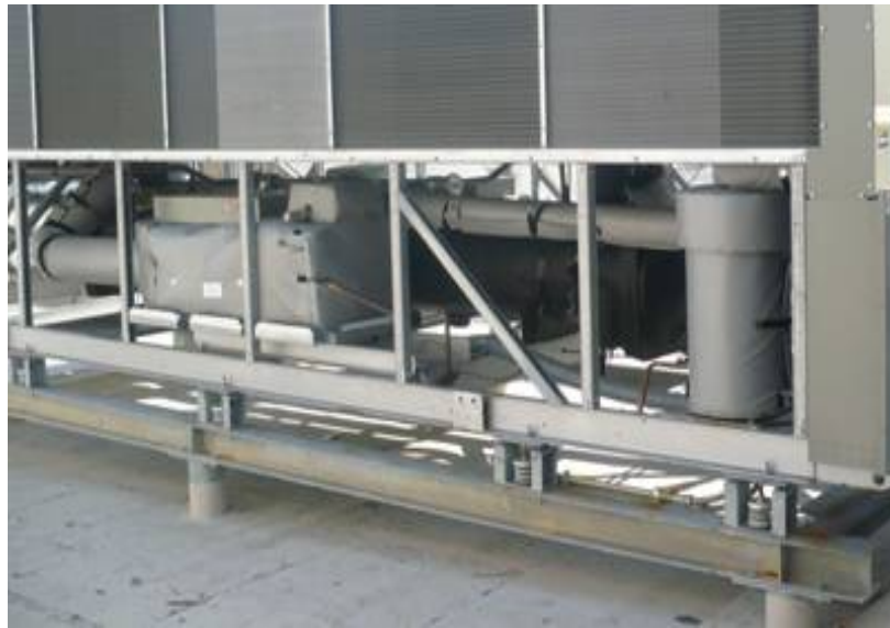
STANDARD™ System on Screw Chiller
