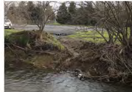
Erosion from stormwater discharge along Rife Run
