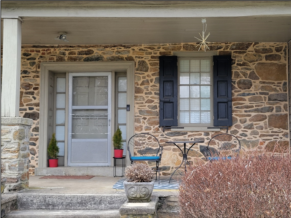
Photo 3. Detail of the first floor of the Miles House, main elevation, facing northwest.
