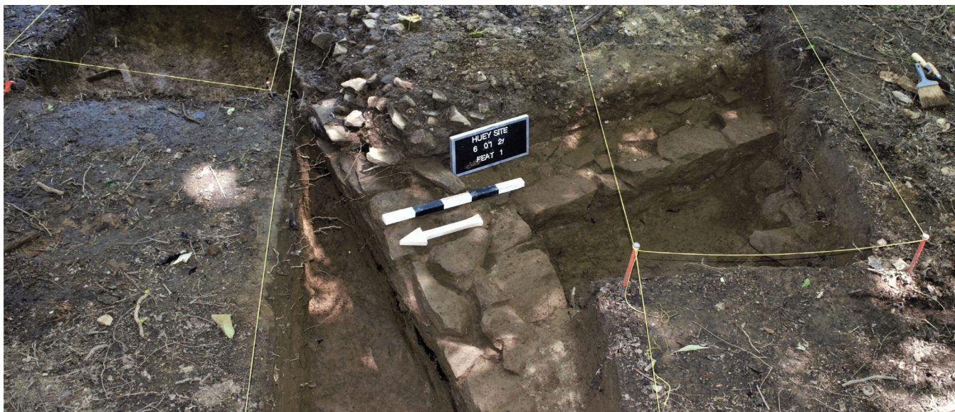
One of the trenches showing a corner of the excavated foundation. Photos for this article were provided by Taria Montes-Rivera.
