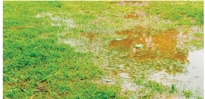
Failed Septic Drain Field
