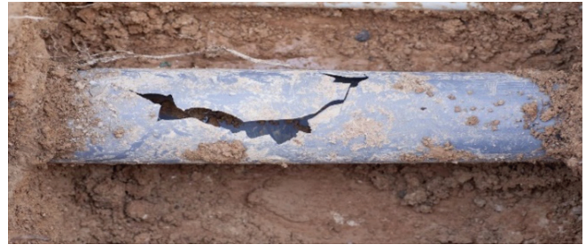
A Ruptured Septic Pipe
