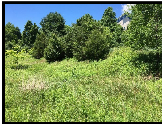
Figure 4: Overall View of Simon and Jude Dry Extended Detention Basin
