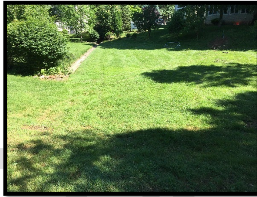
Figure 5: Overall View of Kolbe Lane Dry Extended Detention Basin
