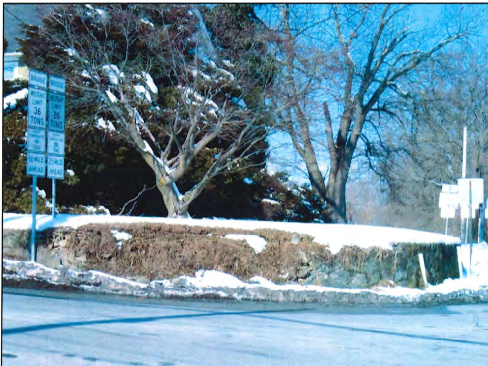
Photo 15 – Stone retaining wall at southeast corner of SR 202 and SR 926, looking northwest
